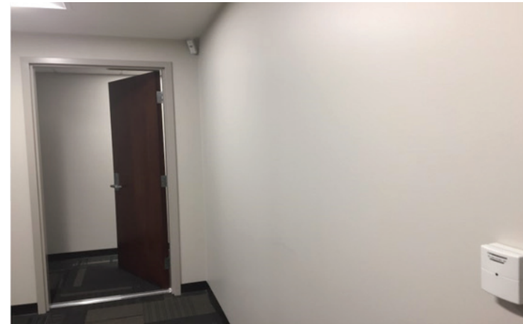
Dual Camera Configuration with PIR Sensor and Thermostat Camera
